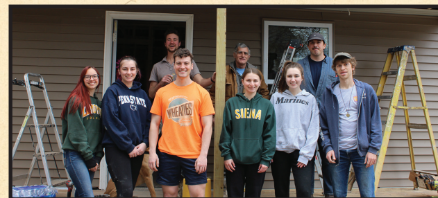
Le Moyne College's Dolphins for Humanity helped place concrete, haul stone, and install soffit at our Ostrander property.
